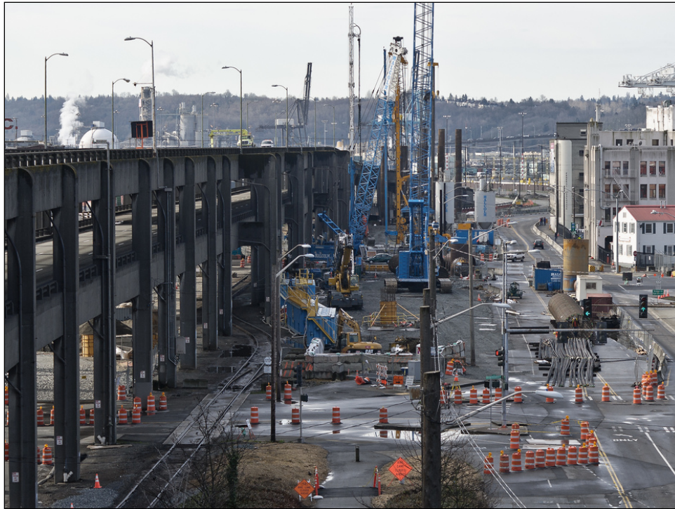
This photos shows the proximity of new construction to the existing viaduct Shaft drilling, pile driving, and ground improvement work are adjacent
